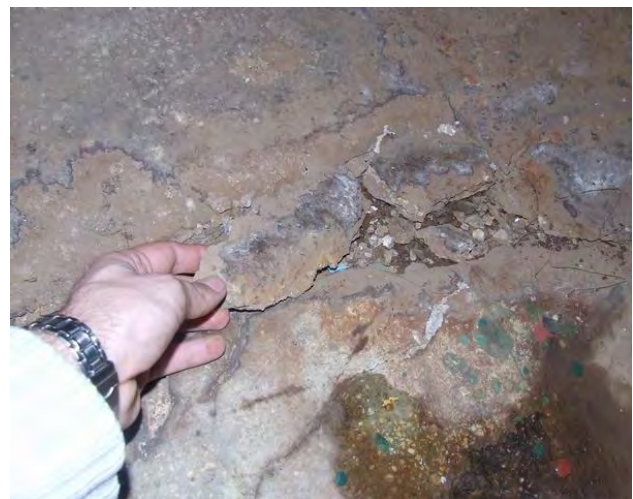
Fig. 3. Detachment of concrete
