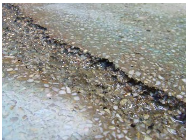
Fig. 1 Corroded area of the concrete floor and exposed rebar in an indoor swimming pool
