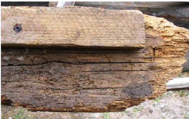
Fig. 1. Damaged ceiling beam end. Wood decomposition due to fungi
