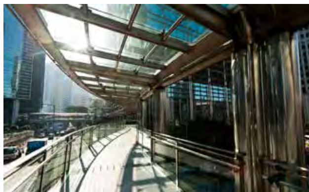
Fig. 3. Footbridge in Cheung Kong Center, Hong Kong [9] Rys. 3. Kładka dla pieszych w Cheung Kong Center, Hong Kong [9]
